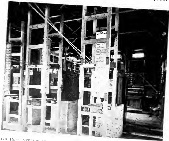
FIG. 16.—INTERIOR OF SUB-STATION, SHOWING LIGHTNING ARRESTERS, ETC.
